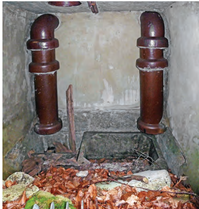
Ventilation pipes near tunnel exit
